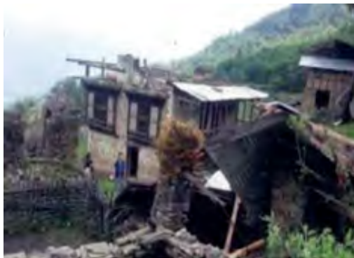
Damage caused by windstorm
