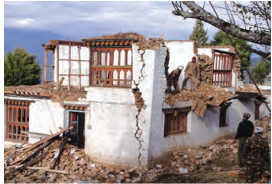
Figure 14.2: Aftermath of Earthquake
