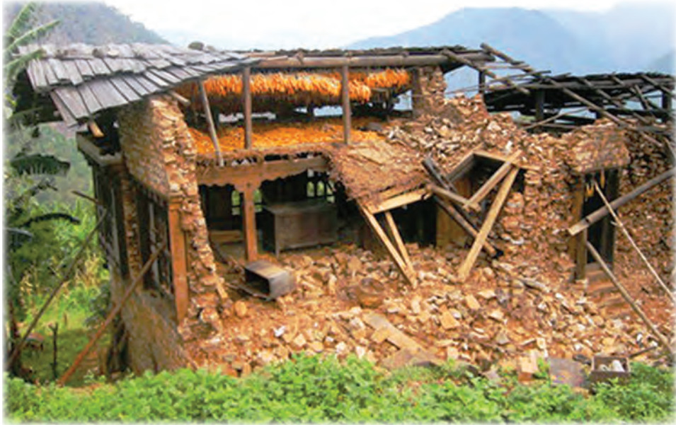
Fig 14.2 Damage by earthquake
