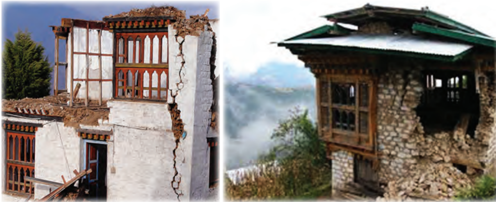
Figure 5.6 Effects of Earthquake in Bhutan
