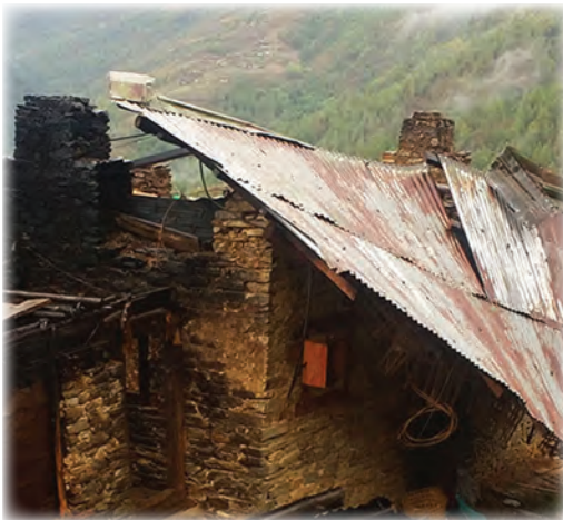
Figure 14.4(a) House damaged by windstrom
