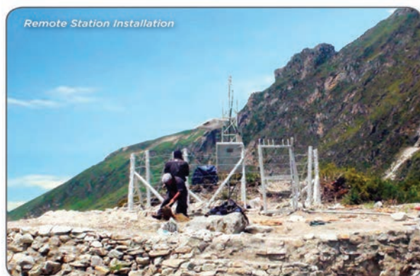
Figure 14.13: Flood monitoring station
