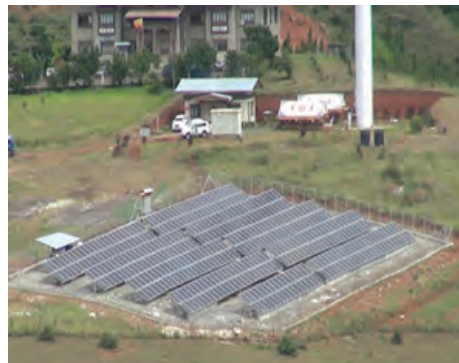
Fig. 11.1 Solar PV plant (180 kW) at Rubesa, Wangdue
